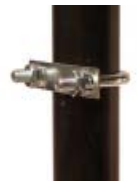
Supplied "U" Bolt on Pole
