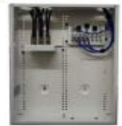
Structured Wiring Panel
