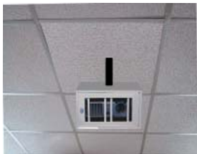
The Pole Mounted Enclosure installed below the Ceiling Tiles
