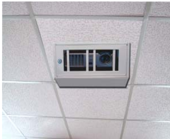
Locking Projector Enclosure mounted flush with the Ceiling Tiles
